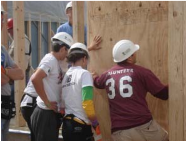
(From left) Banderanko, Centrowitz and Culp work to put up a wall on the construction site. Photo by Ellie Storck.
